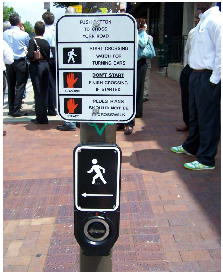
FIGURE B-12: VIBROTACTILE PUSHBUTTONS POINT USERS IN THE SAME DIRECTION AS THE CROSSWALK. (PHOTO CREDIT: TOOLE DESIGN)
